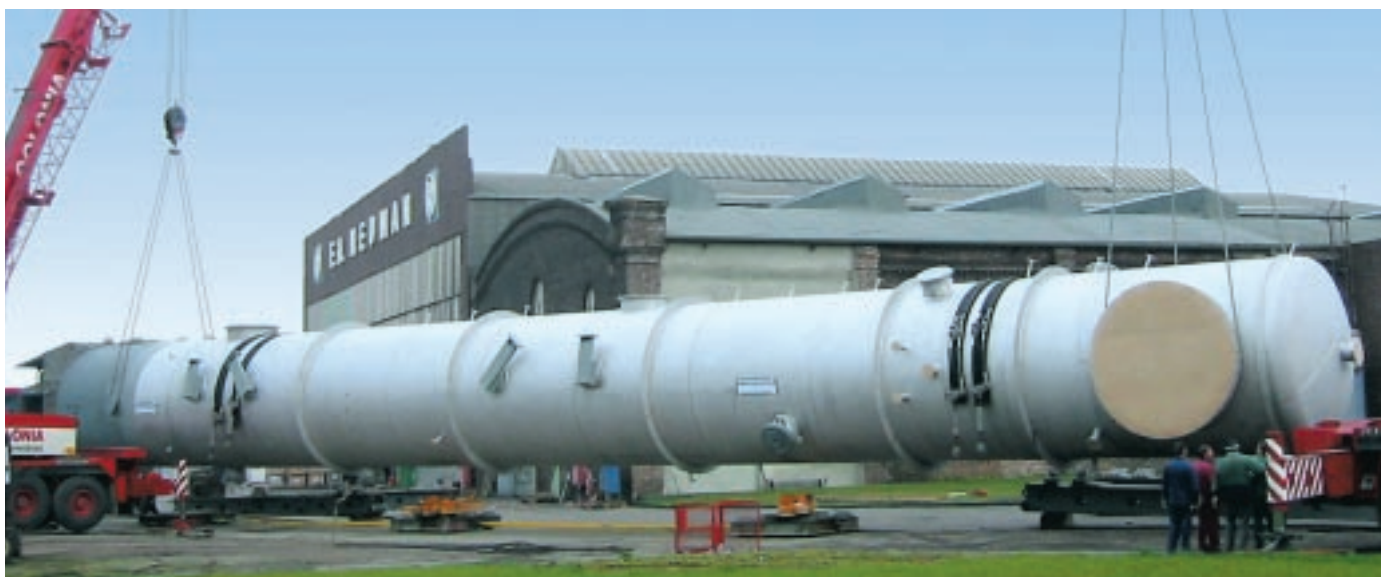
▼ Dividing wall column DN 3600
